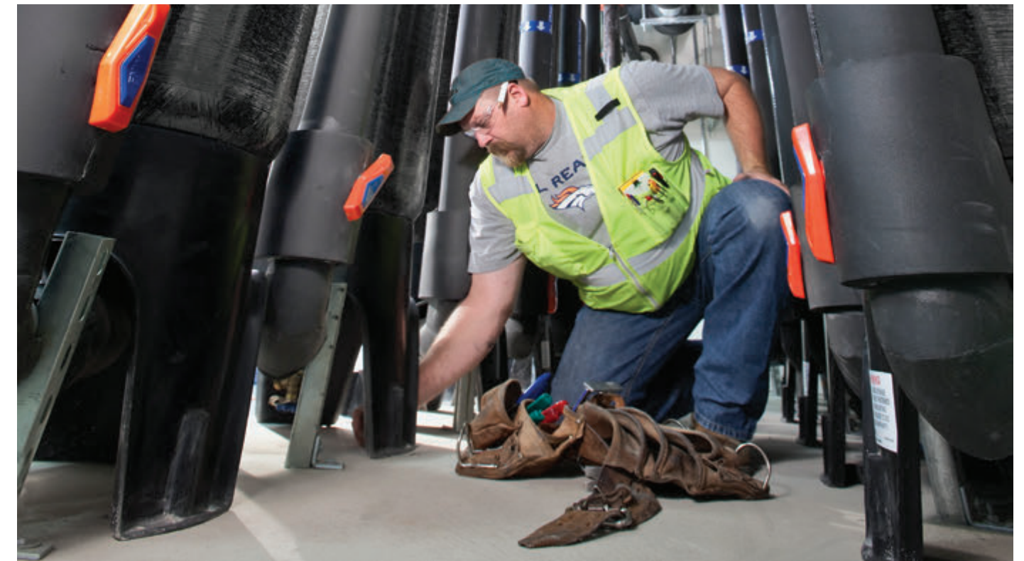
A Watts OneFlow® antiscale system installation.
