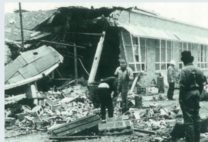
George Horne also constructed dramatic presentations of mounting pressure and its consequent explosions, displaying the necessity for T&P valves.
